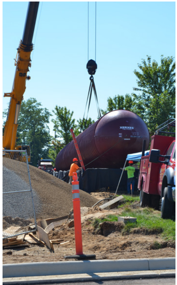
Workers place one of the underground gas tanks at the Pit Stop.
