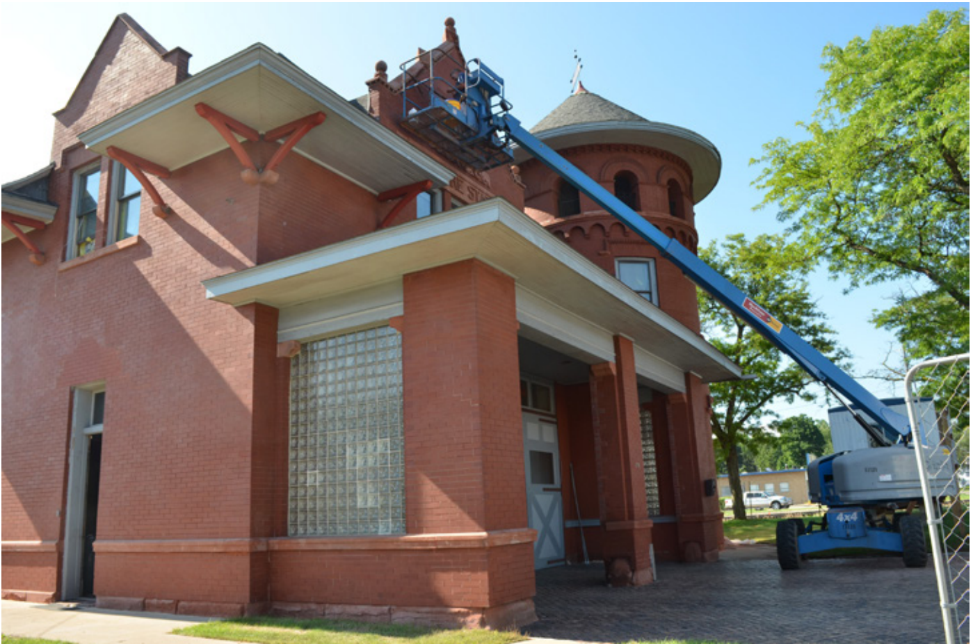
The exterior of the historic fire station in Battle Creek gets power washed
