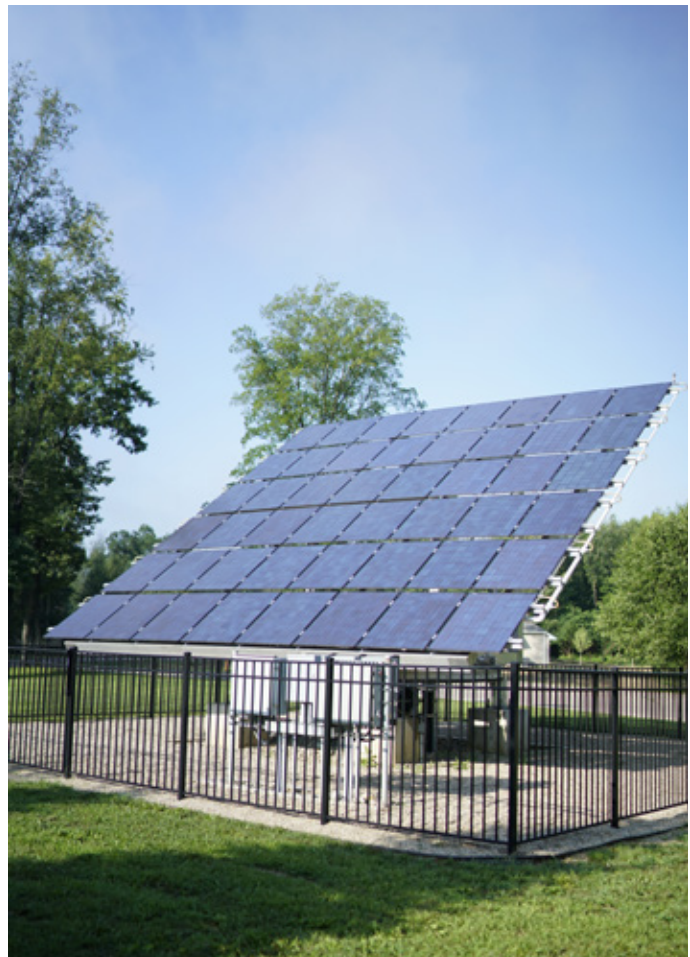
The Skasge Power, LLC solar array warms the water for the Pine Creek Community Center.
