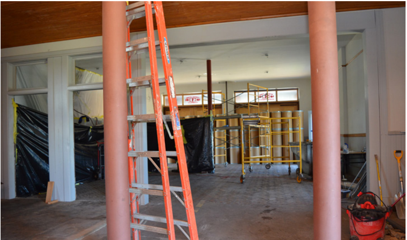
Demolition and reconstruction are underway in the interior of the old fire station to make way for a restaurant and food pantry.
